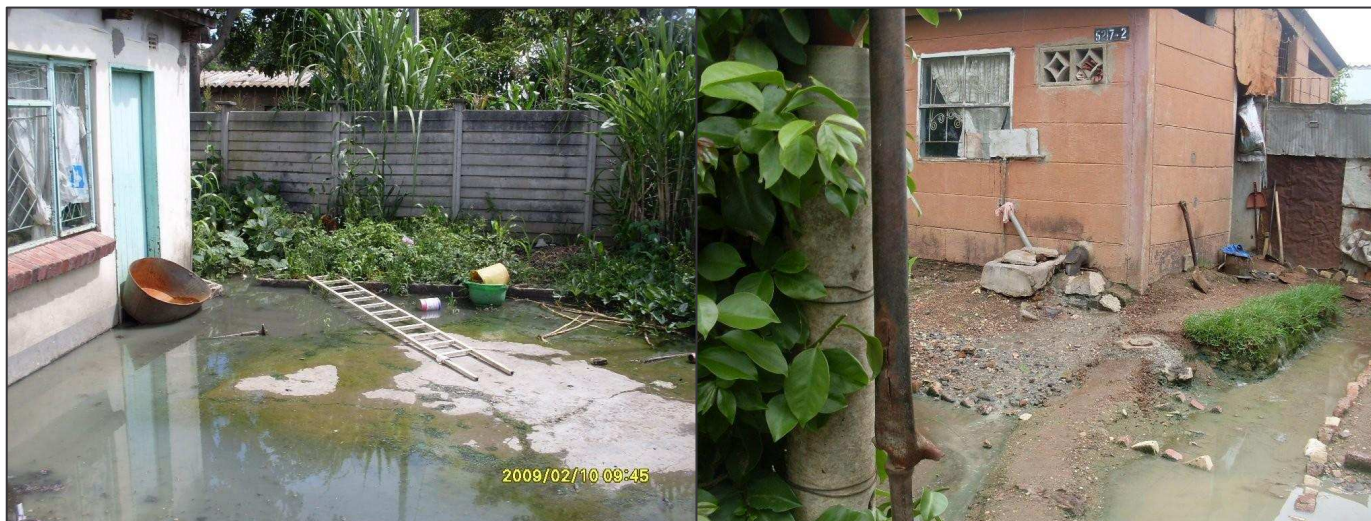
Raw sewage from burst sewer pipes flows outside homes in Mkoba and Athlone, Gweru Photos courtesy of Zimbabwe Lawyers for Human Rights
