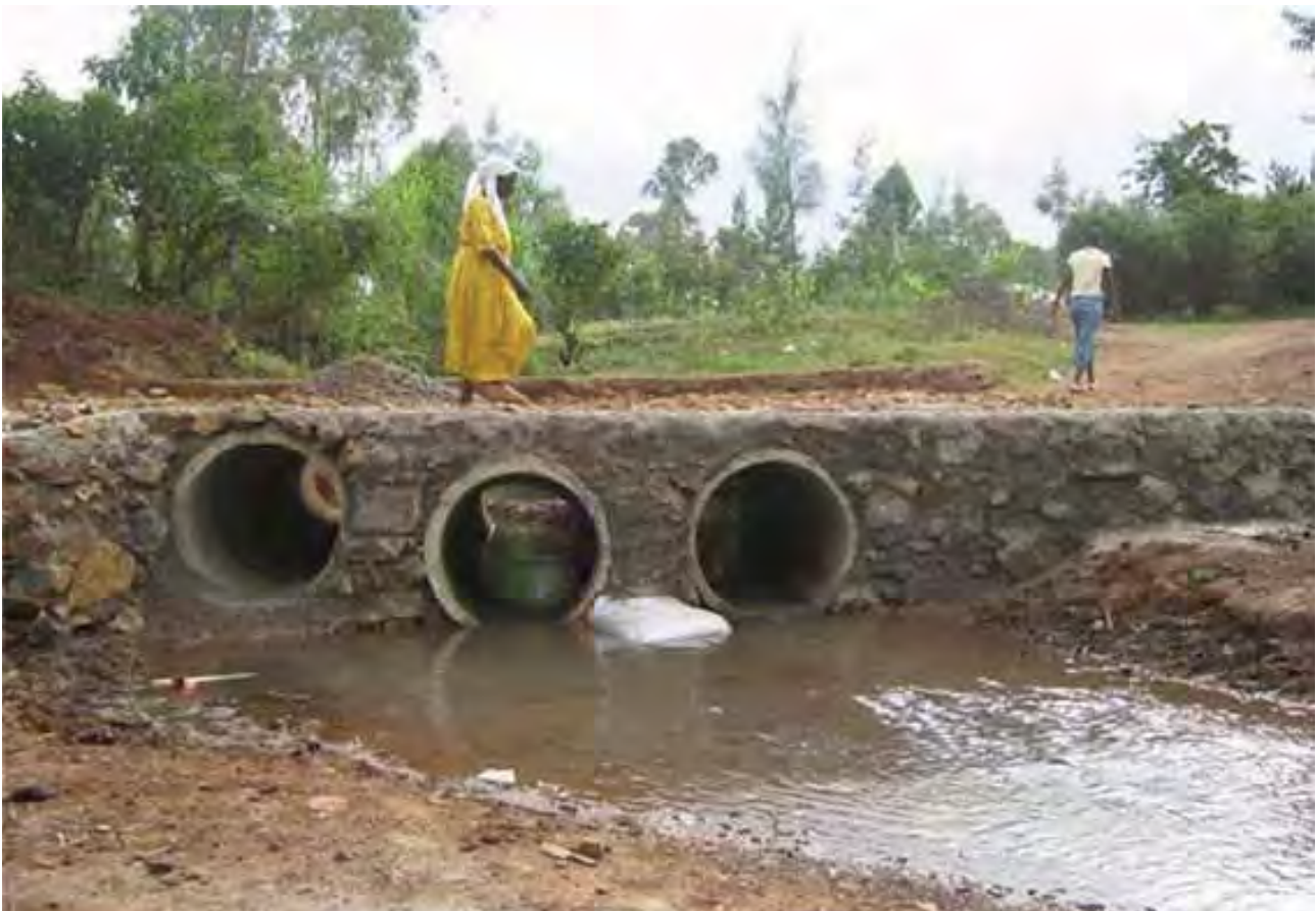
The community built a bridge for people to access the local market, Kasipul, Kenya
